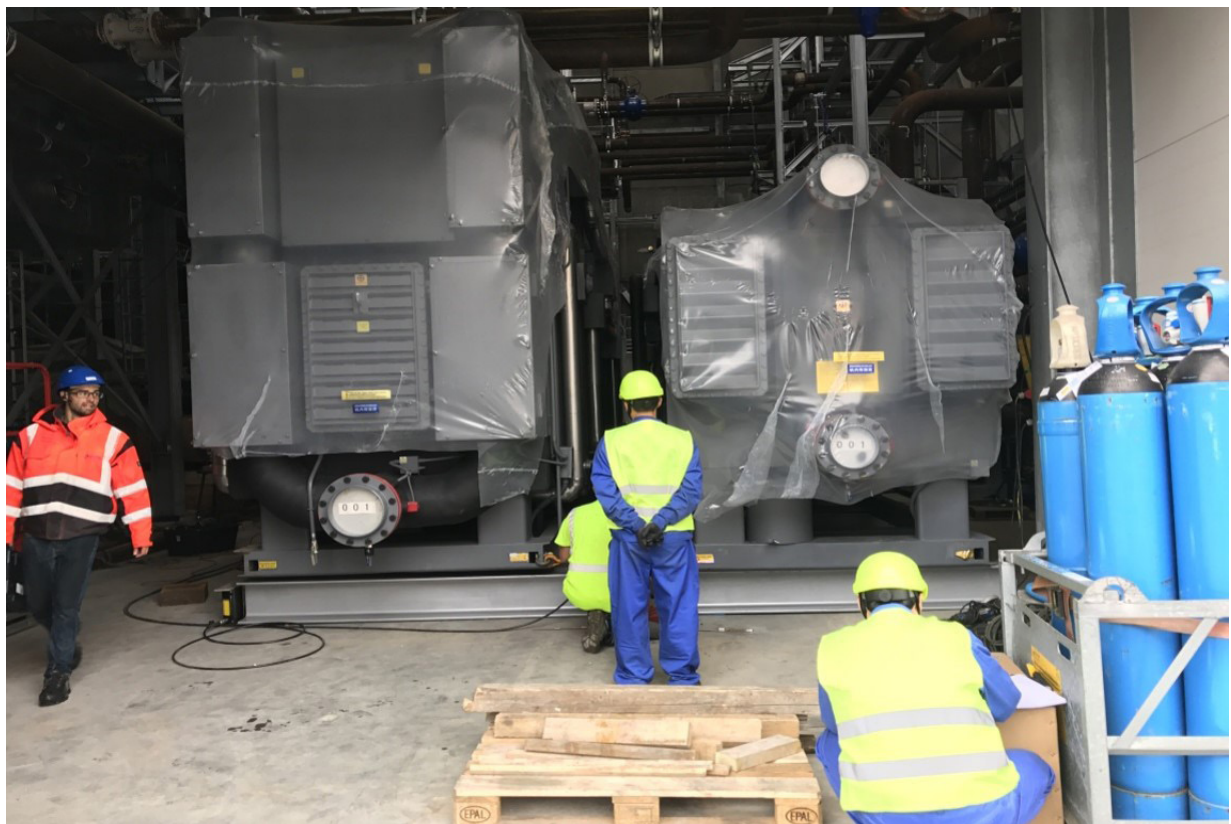
Grenaa District Heating heat pump machine room 格雷诺区域供暖机房
