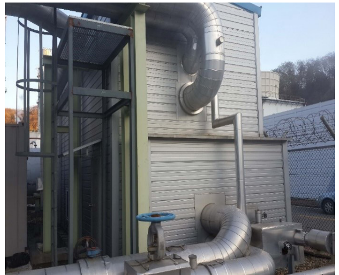
Machine room of Bundang Power Plant heat pump 盆塘电厂热泵机房
