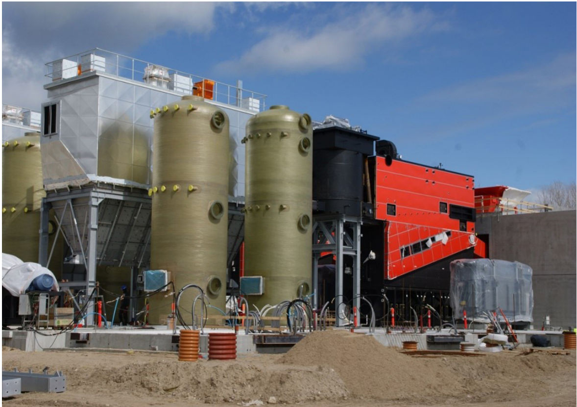
Grenaa District Heating heat pump machine room 格雷诺区域供暖机房外景
