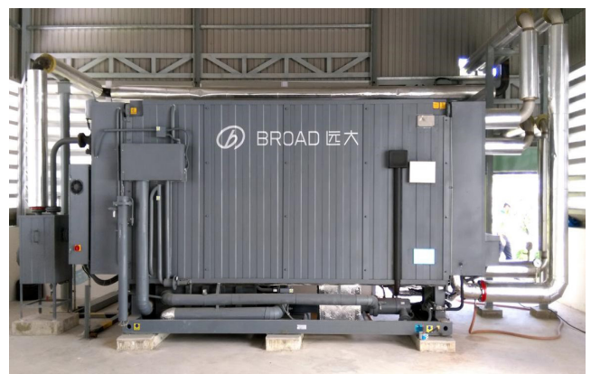
Machine room 热泵机房
